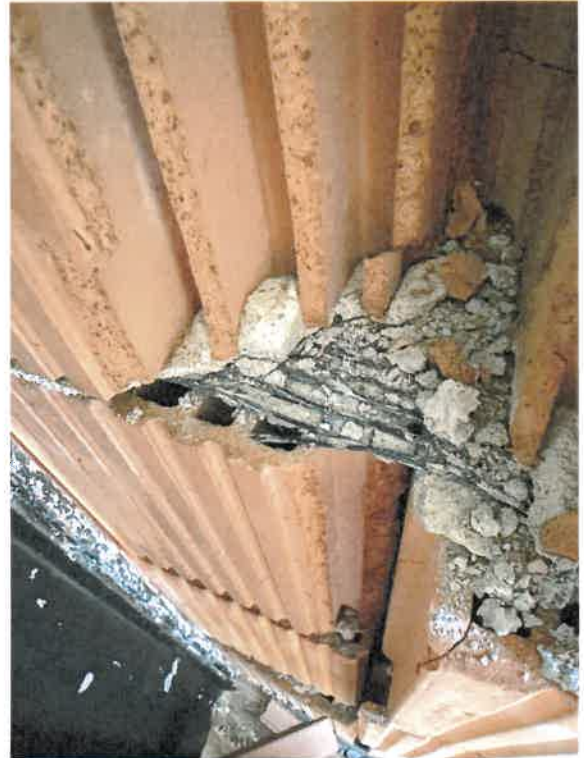
Figure 15 - Detail of reinforcement stretching and tearing
